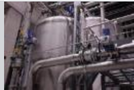
Control valve solutions
